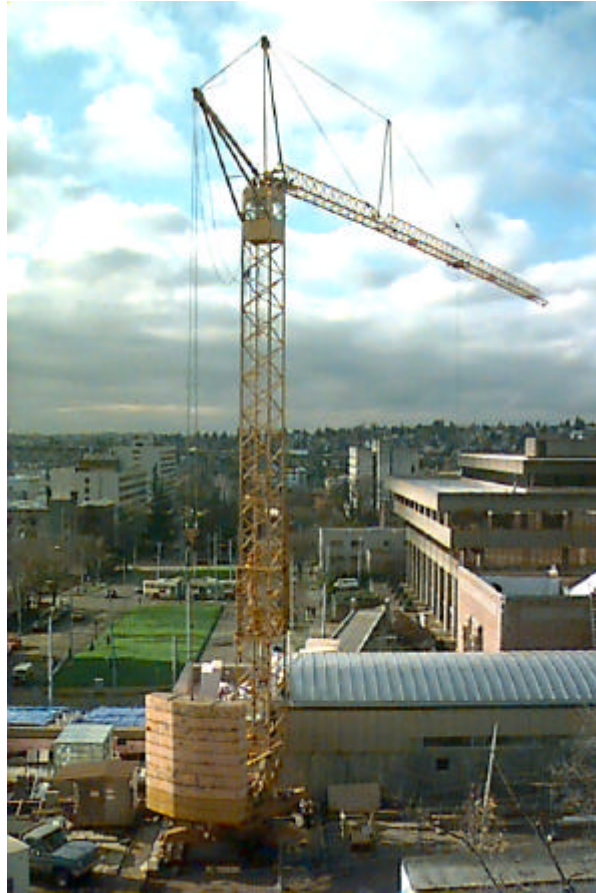
Figure 6. Images taken from neighboring buildings at regular intervals provide an excellent record of project progress.
