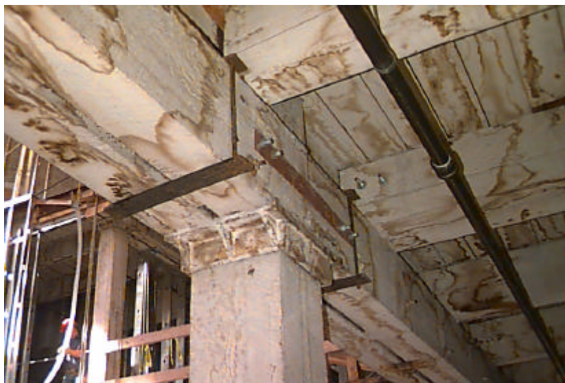
Figure 4. Close-up images of building details can be placed on Internet sites and viewed instantly by project players in remote locations.
