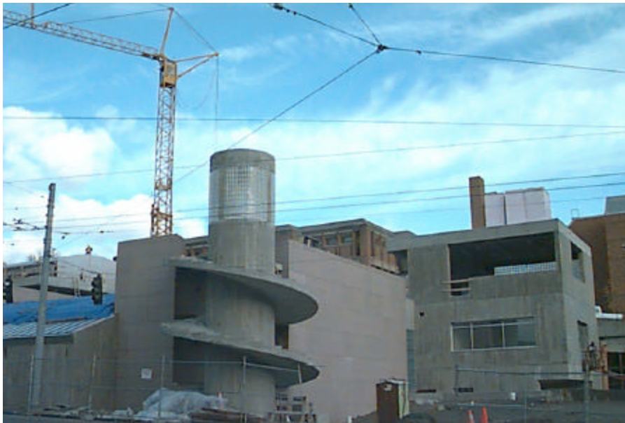
Figure 3. Progress image of the Henry Art Gallery Expansion at the University of Washington Campus, Seattle, WA.
